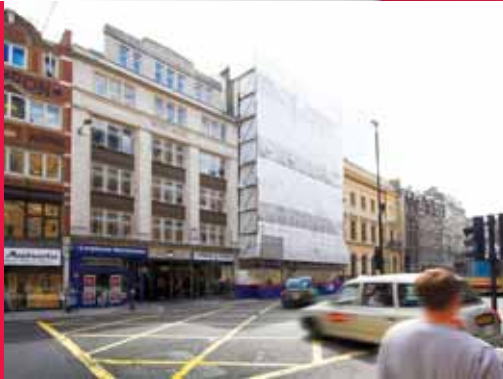
Strengthening of concrete floor slabs on five floors for Vinci UK Fleet Street, London, UK
