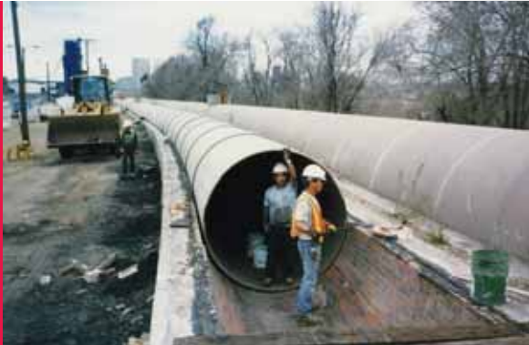
Structural retrofit with TFS® of Denver Water. The best option for a completely trenchless renewal of this magnitude.
