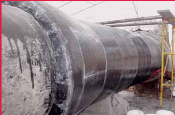
Emergency Rehabilitation and Repair of reinforced concrete pipeline section of Water Supply (EYATH) , Thessaloniki, Greece
