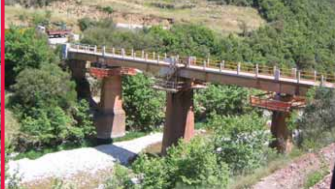
Structural Upgrade and increase of the loading capacity of Evinos river Bridge at Grevena, Greece
