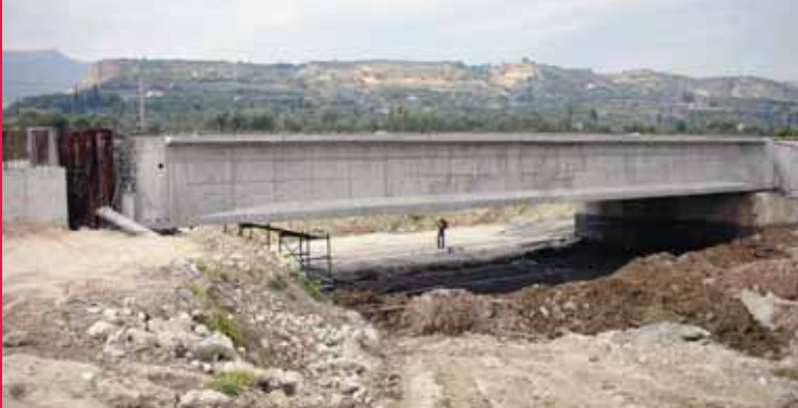
Emergency Structural repair of Railway Bridge , of Hellenic Railway Organisation, Kiato, Greece
